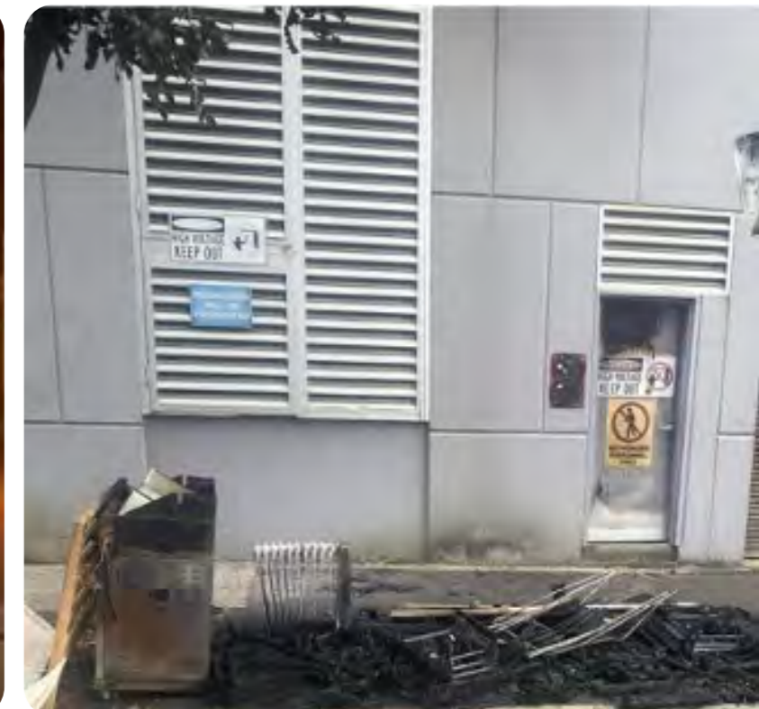
Fire and its aftermath at Metro Village Rosebery
